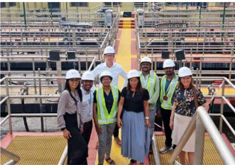
IVL visiting the treatment plant on the Mithi River in Mumbai, India.
